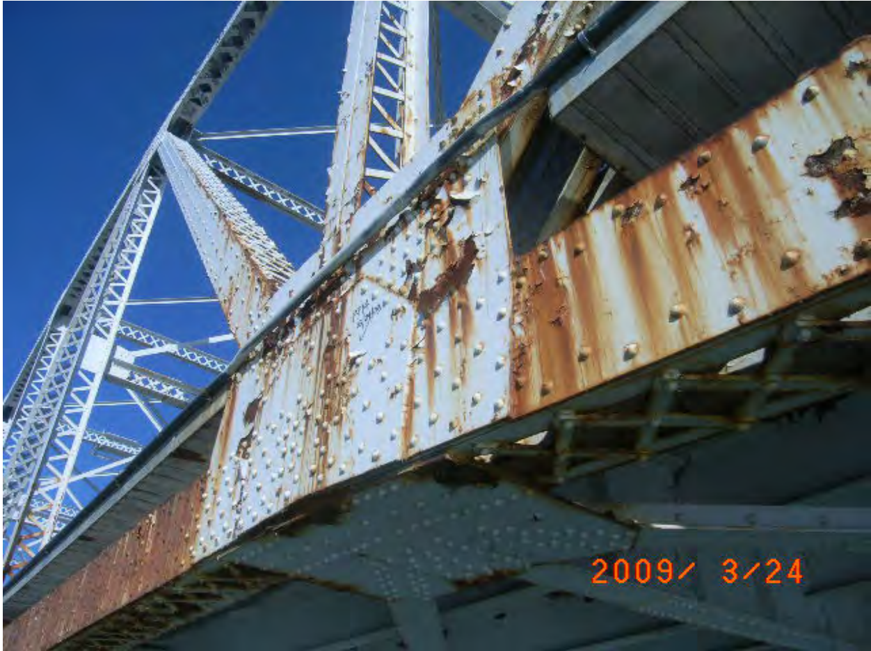
Figure 113. Span 7 lower chord connection at L14.
