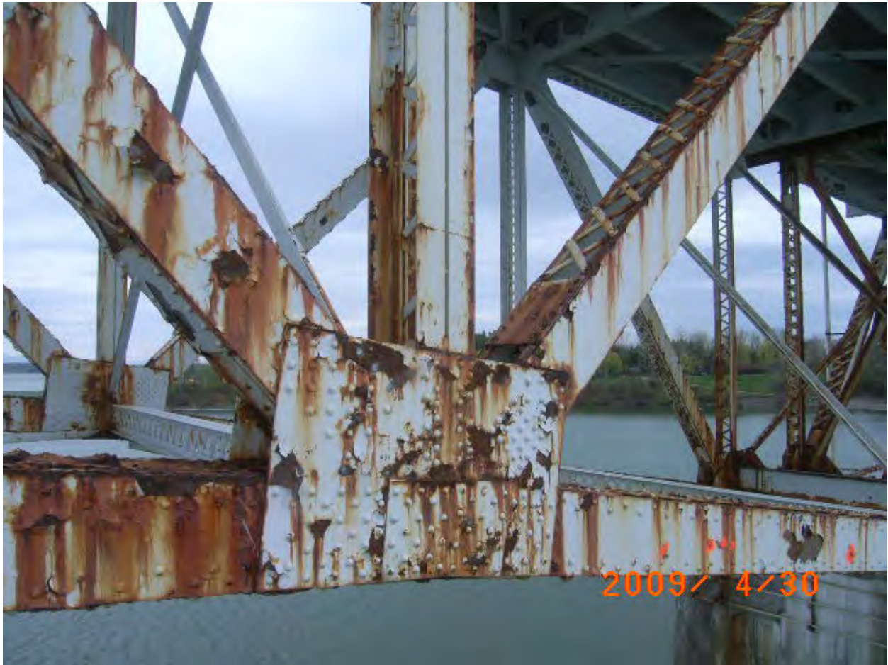
Figure 122. Span 6 lower chord connection at L02.
